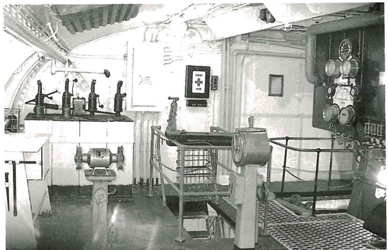
The upper level of the engine room.
