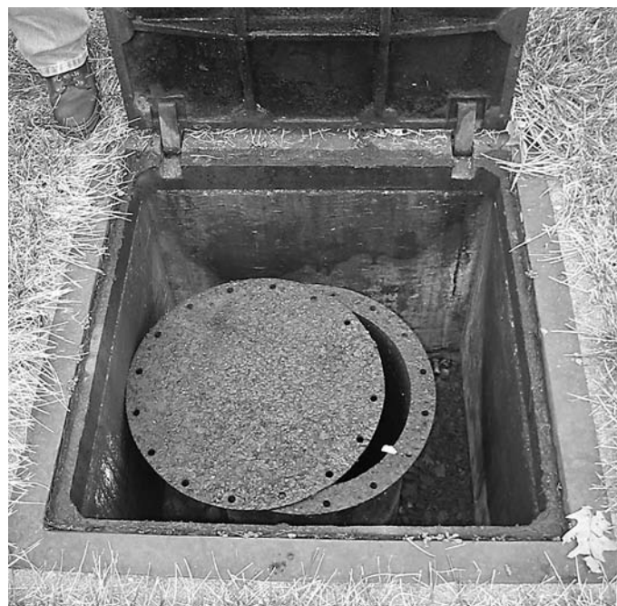
Pump-out port for separator tank.
