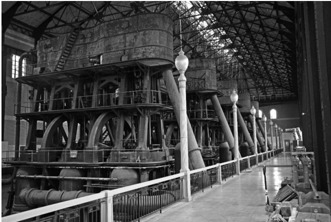
Colonel Ward Pumping Station Porter Avenue Buffalo
