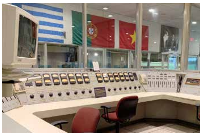
Control room at the VOA Bethany Relay Station.
