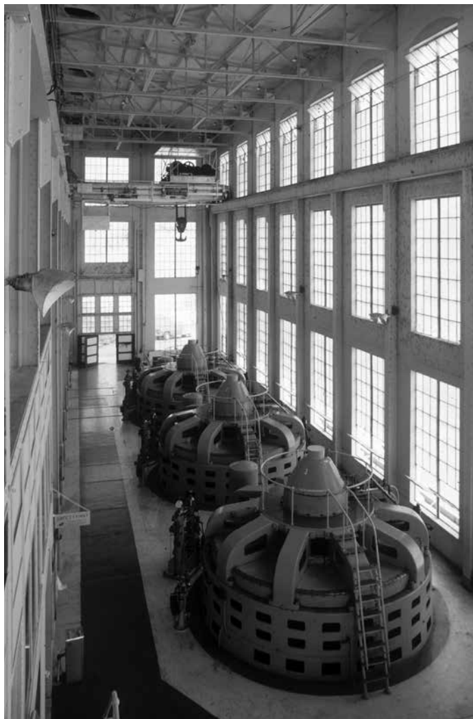
The interior of the Ryan Powerhouse features vertical-shaft turbine-generator units.
