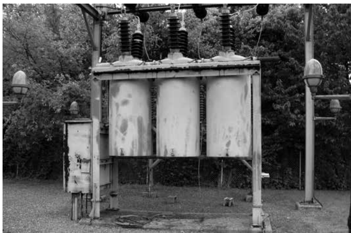
Large oil circuit breakers at a 1940s industrial plant located in Pennsylvania. The manufacturer's plate states that the breakers were manufactured in 1959, and each contained 285 gallons of oil. Note the taps for draining the oil. Highly suspect for PCBs.
