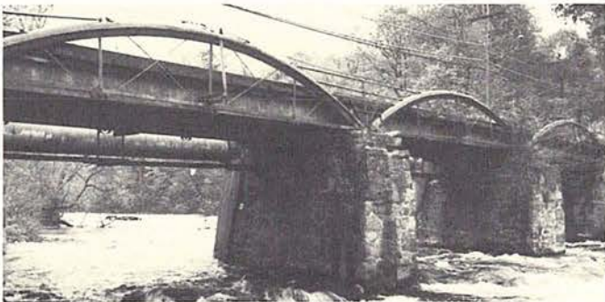
Tioronda Bridge. The deck today is carried by concrete girders, the trusses structurally inactive.
