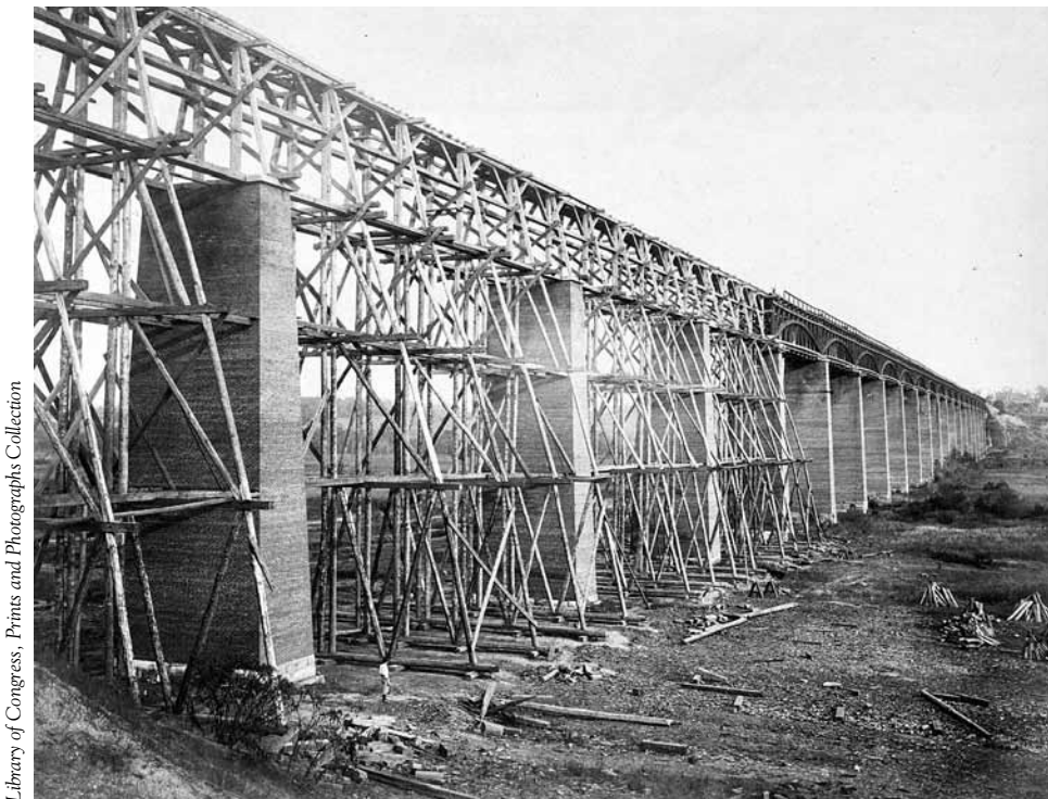
High Bridge, ca. 1865. Photograph by Timothy H. O'Sullivan, following the Battle of High Bridge, showing the reconstruction of four spans damaged during the battle.
